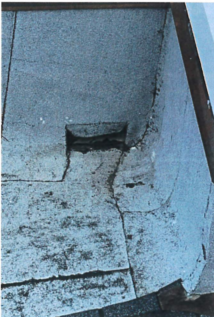
4 Scuttle hole to be repaired.
